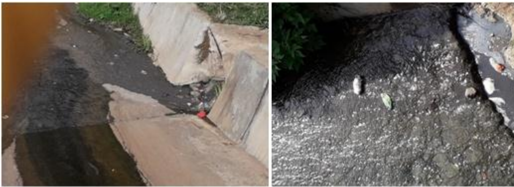
Figure 1.1: Raw sewage leaking directly into Iini Stream, in Machakos town (Location -1.5225467 and 37.2713401)
